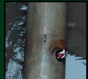
Right: A special "wrench-bob" was used to perfectly locate what is to become the center of the new manhole.
