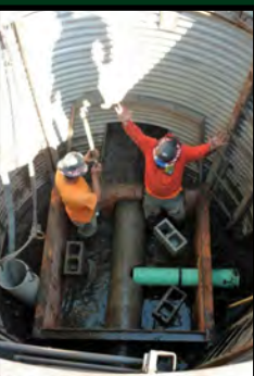
Left: Finally the new 8" diameter pipe was perfectly set for alignment and grade—as Karl celebrates success!
