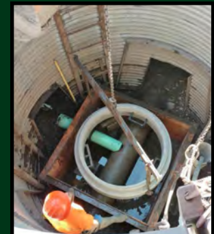
Right: A 1' ring is then set into place being supported by concrete blocks.
